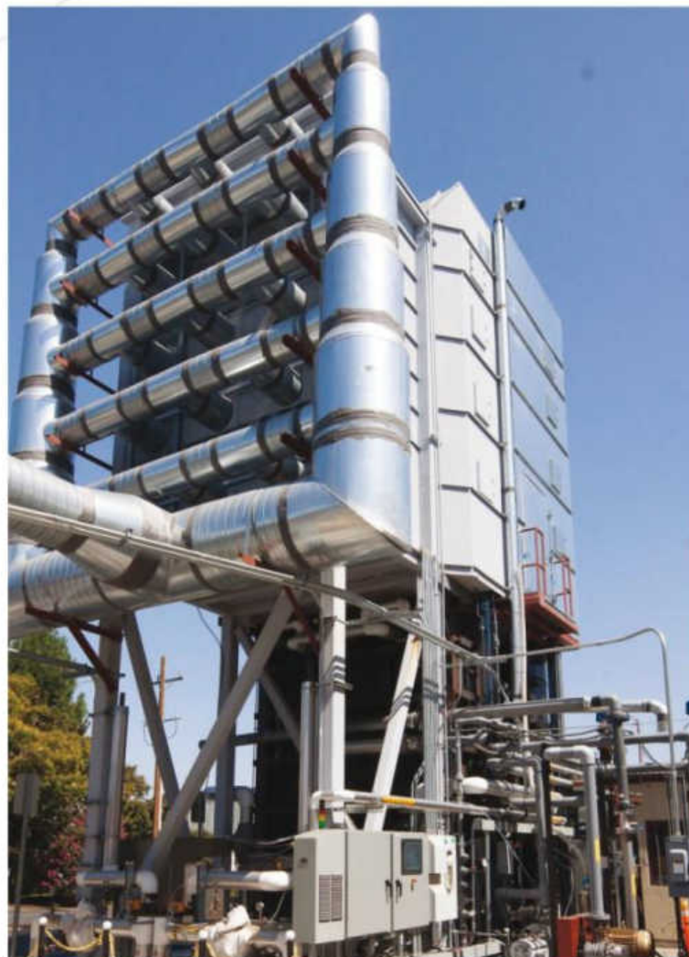
Global Thermostat's test unit at SRI International's Menlo Park campus extracts carbon dioxide from the fumes of SRI's natural-gas-driven power plant.
